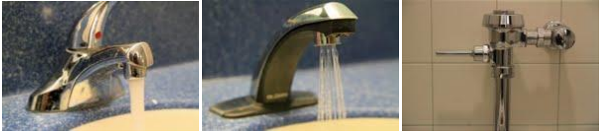
Figures 4, 5, & 6. Figure 4 shows a regular flowing faucet, which are the faucets implemented in Mosher-Jordan's Residential bathrooms. Figure 5 shows a low-flow faucet, that is also a sensor faucet, which are implemented in the non-residential bathrooms at Mosher-Jordan. Figure 6 shows the standard toilet flush/valve that has been implemented in residential bathrooms. (Source: Elyssa Wiegand)
